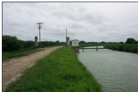
PHOTO 3 PUMP CONTROL PANEL
