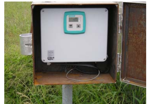
AMR RTU Installed in Metal Vandal Box
