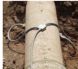
Siemens SONOFLO Ultrasonic Flow Meter 18" Concrete Pipe
