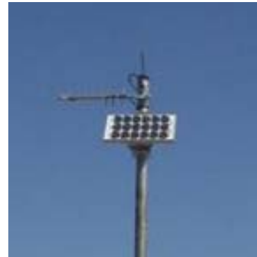
1000 m W — 900 MHz SS Radio for Transmission up to 7 miles with 20 W Solar Panel and Yagi Antenna
